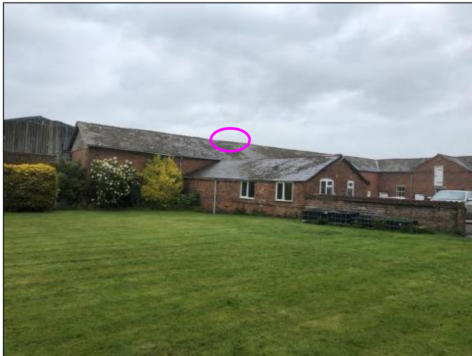
Plate 2 - Emergence area - Emergence of one Brown long-eared bat via a gap at the ridge where it has warped slightly, with commute to the nearby hedgerow headed west. During dusk survey 1.
