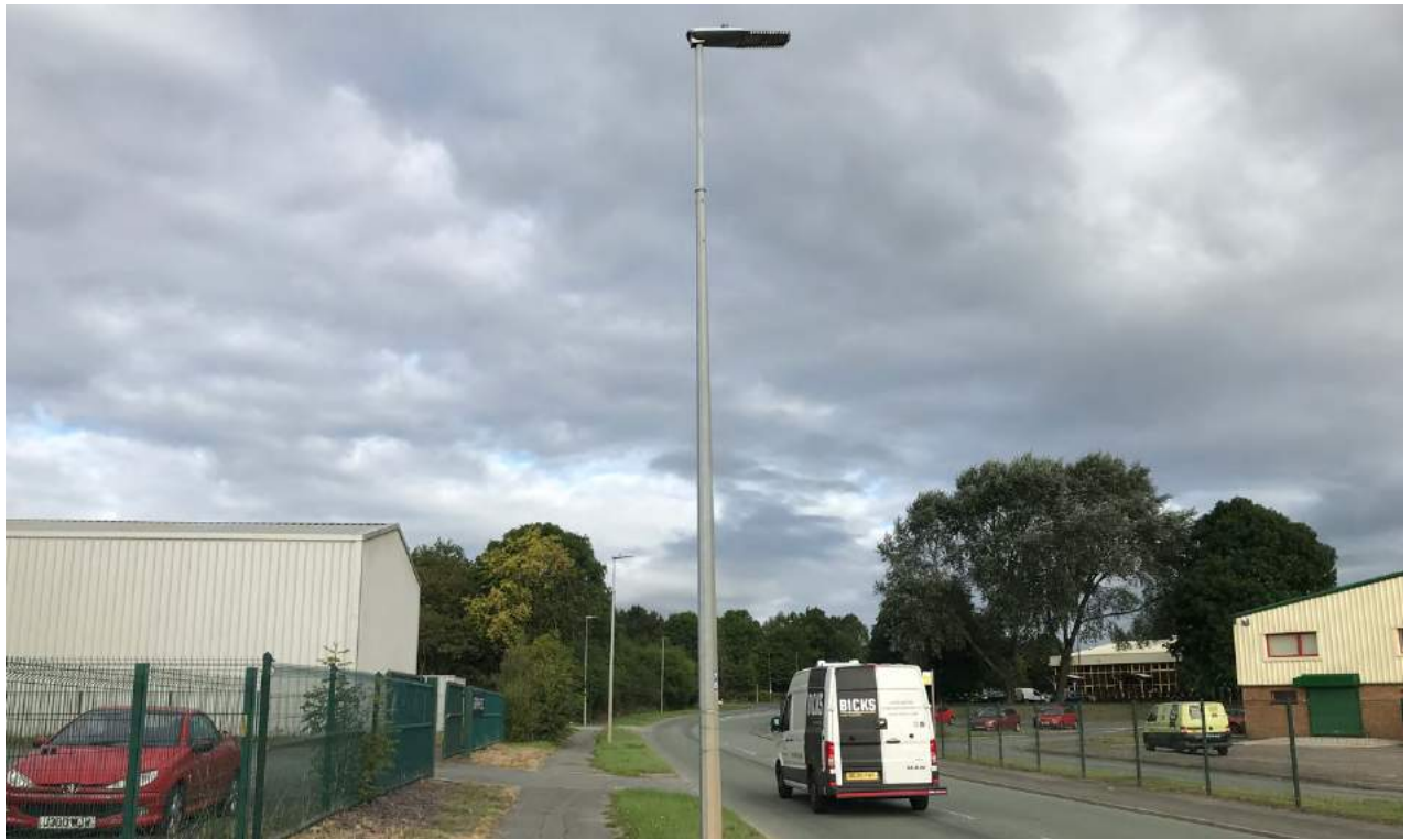
Photograph 2.5 : Coed Aben Road – Street Lighting Columns
