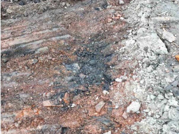
12.04.18 – Minor diesel staining within the made ground.
