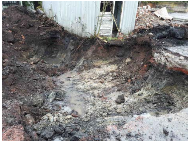
12.04.18 – Pockets of water present within the made ground.
