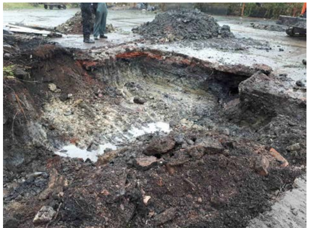
12.04.18 – Visible diesel impacted made ground present to the south of the initial excavation.
