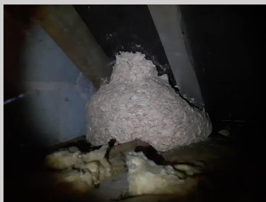
Photograph 2: Wasp nest in smaller roof void
