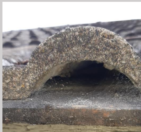
Photograph 12: Cobwebbed damaged tile end
