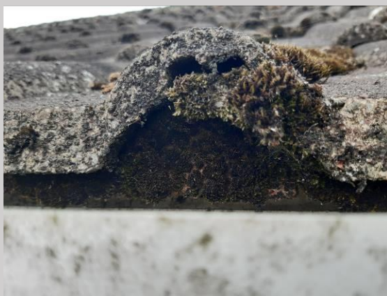
Photograph 9: Damaged but stable tile infill
