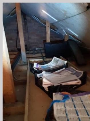
Photograph 6: Broken insulation in larger roof void
