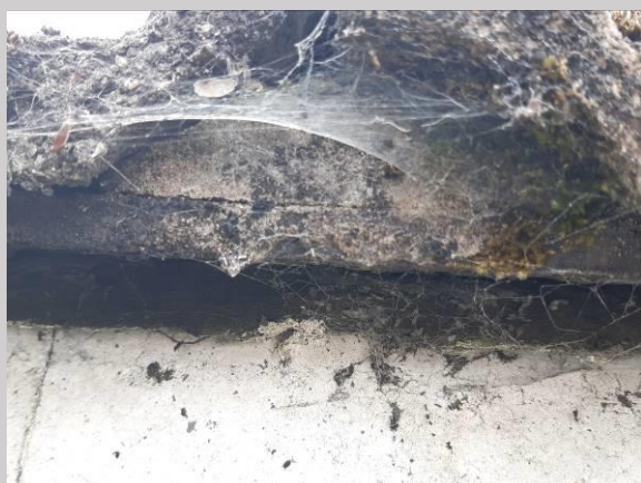
Photograph 11: Cobwebbed stable tile end
