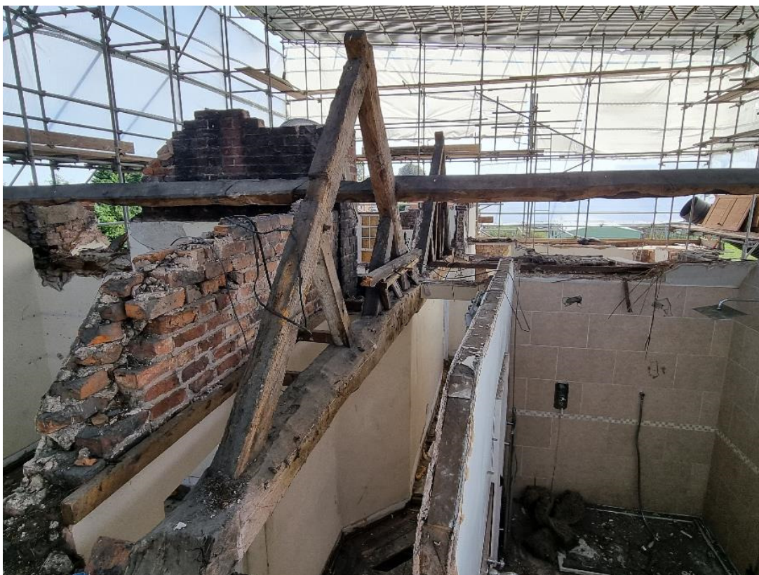
Photo 16: Landing and bathroom with remaining roof trusses, facing south
