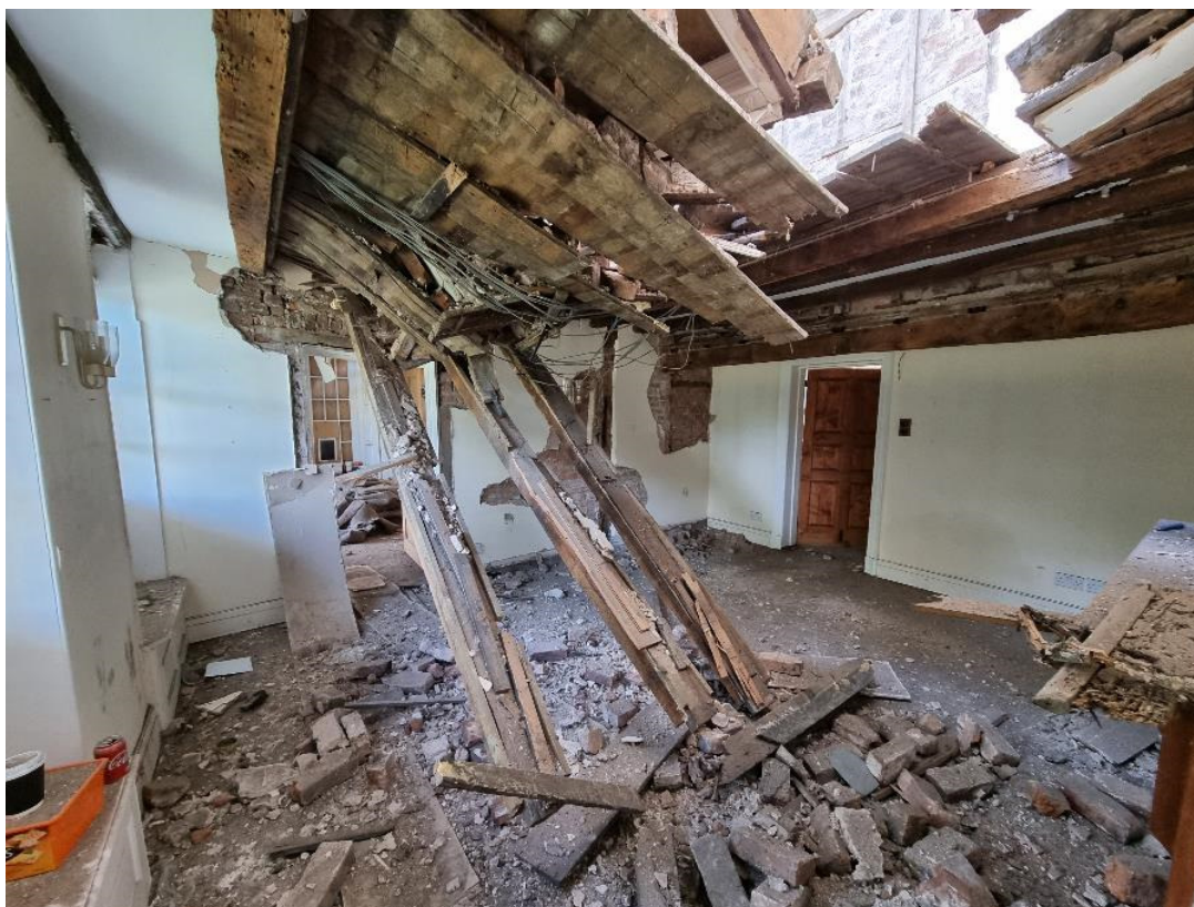
Photo 20: Lounge showing ceiling collapse, view to south west
