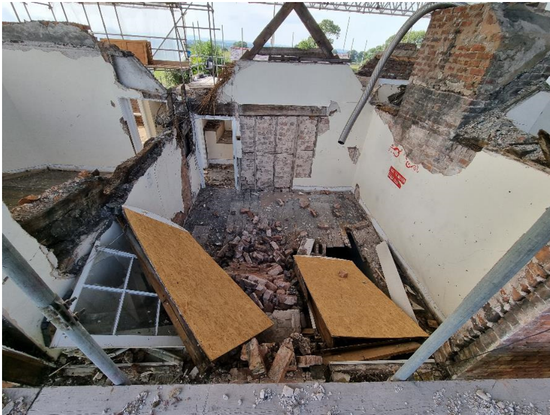
Photo 11: Bedroom 2 facing west through wall collapse
