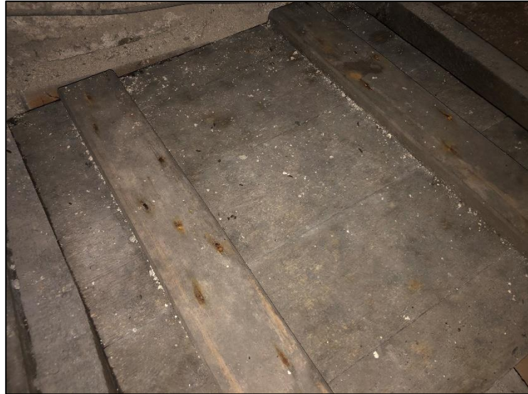
Scattered bat droppings on loft hatch.
