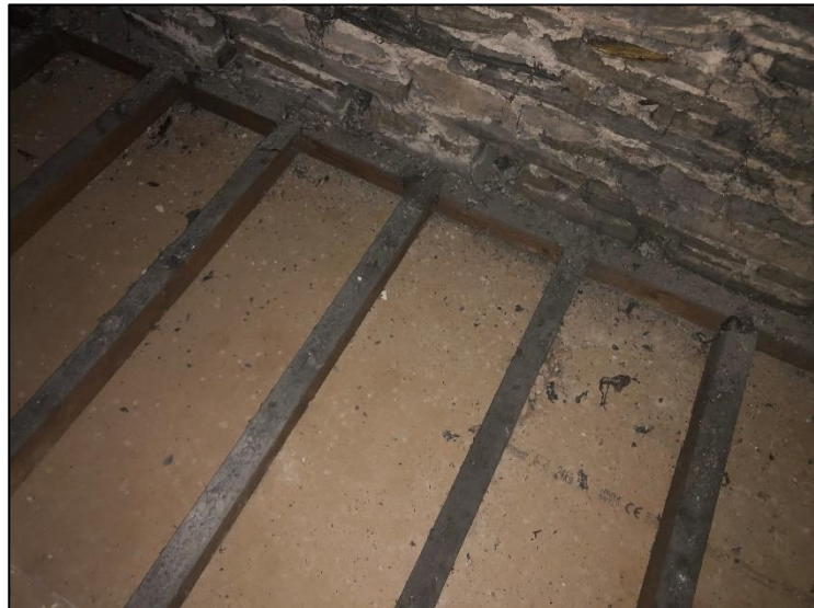
Scattered bat droppings below the gaps in the western gable end.
