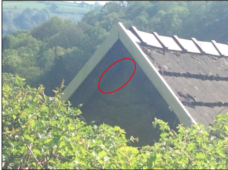
Gaps in the apex below the soffit box on the western gable end.
