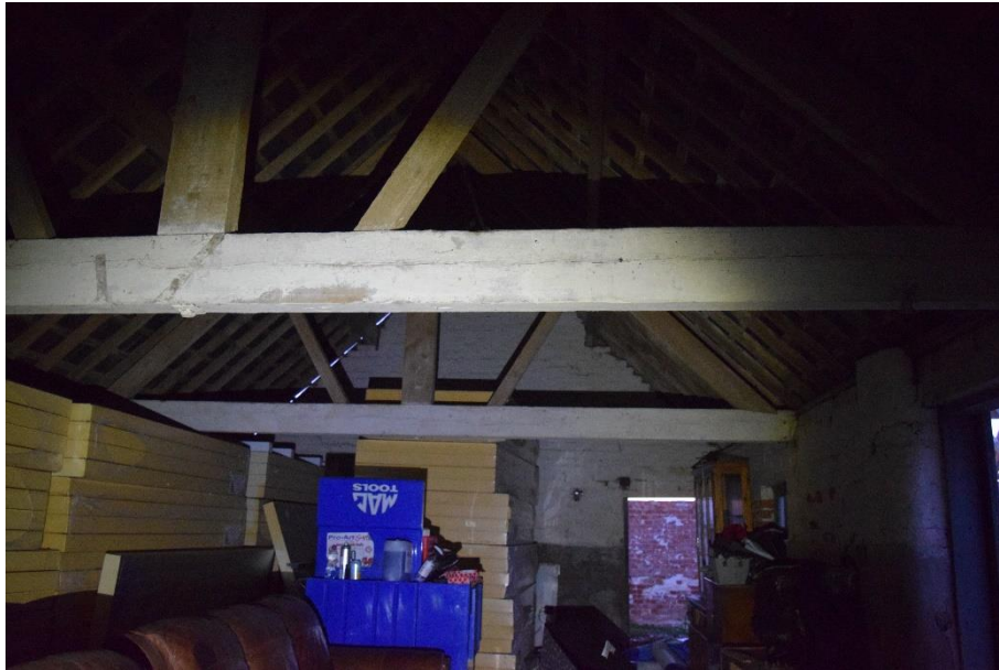
Figure 4.8. Showing gap along western elevation
