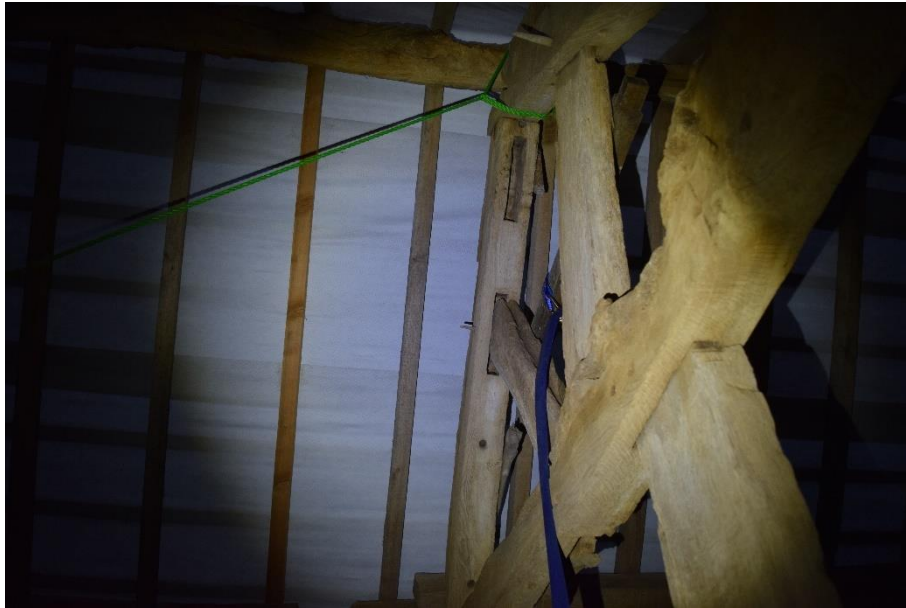
Figure 4.4. Open mortice joint in roof timbers
