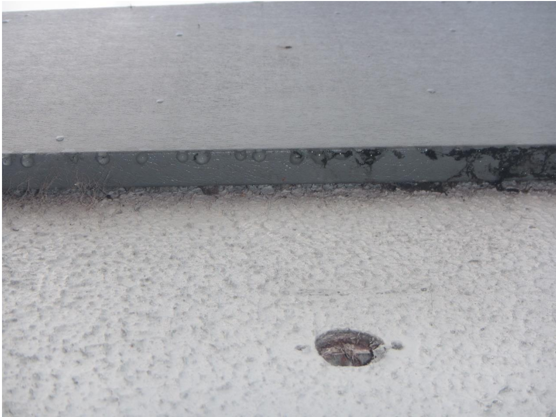
Photograph 13 – Lifted barge board on the northern aspect of Building A
