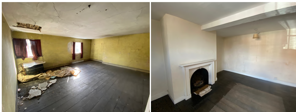
Second floor room with failing ceiling and bedroom
