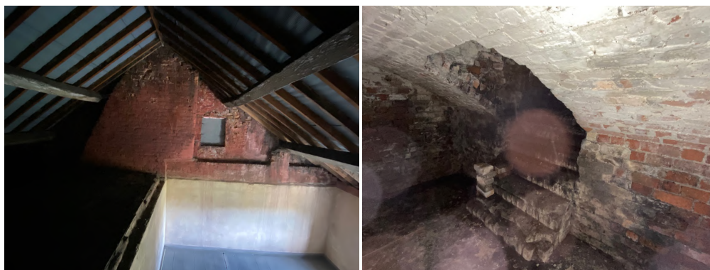
Second floor room with lost ceiling (viewed from attic) and cellar
