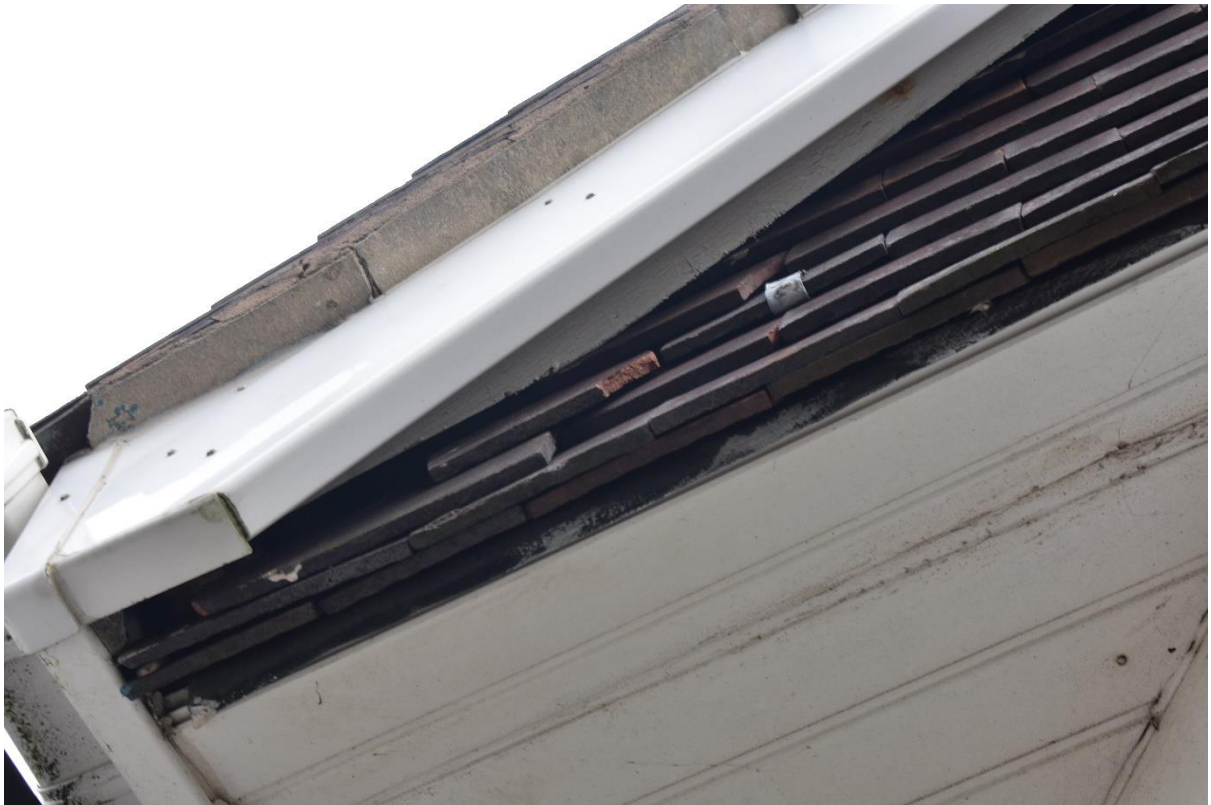
Figure 3.6: The gaps present on the hanging tiles fitted onto the dormer window.
