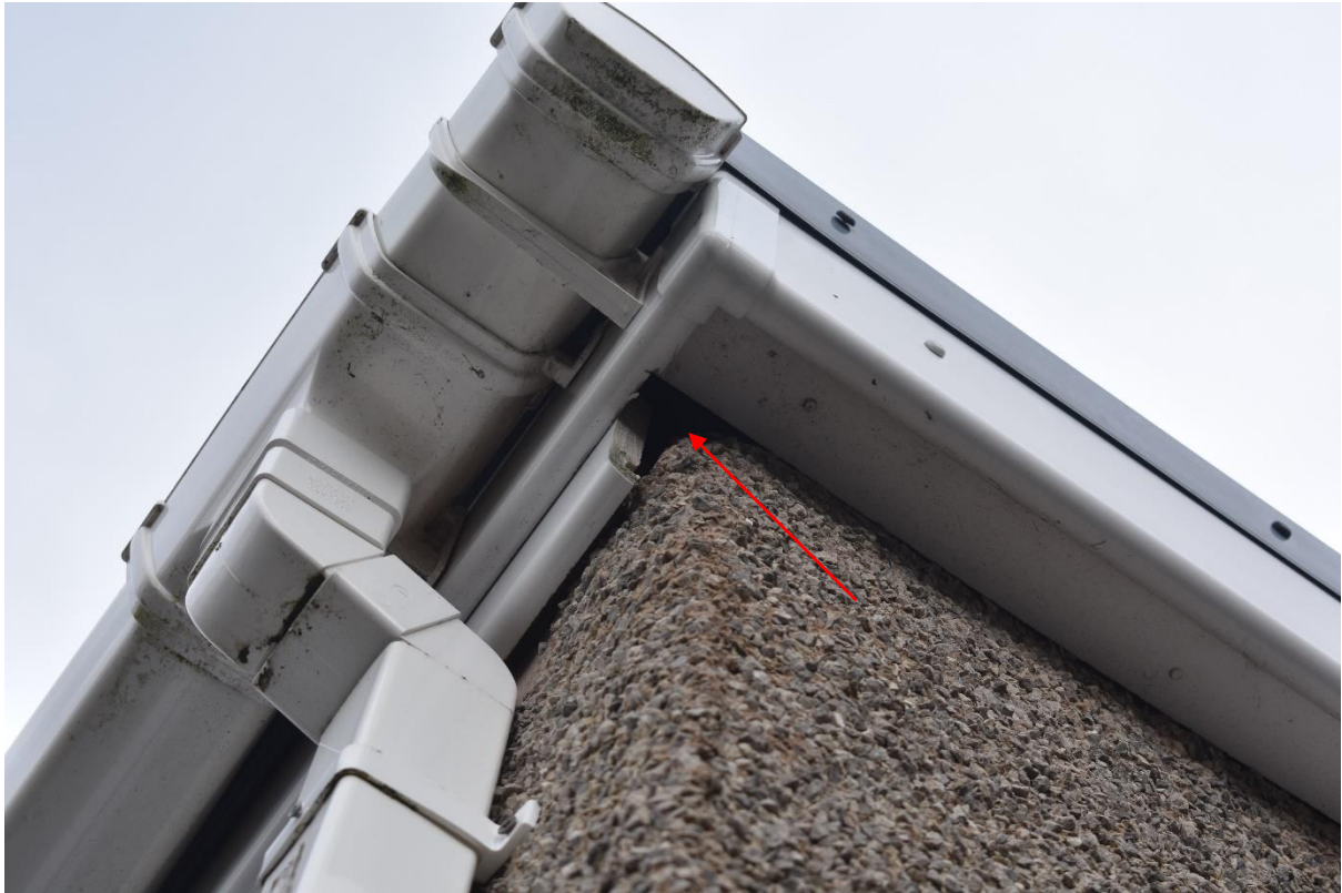
Figure 3.7: The single gap present between the soffits and the wall of the dwelling.
