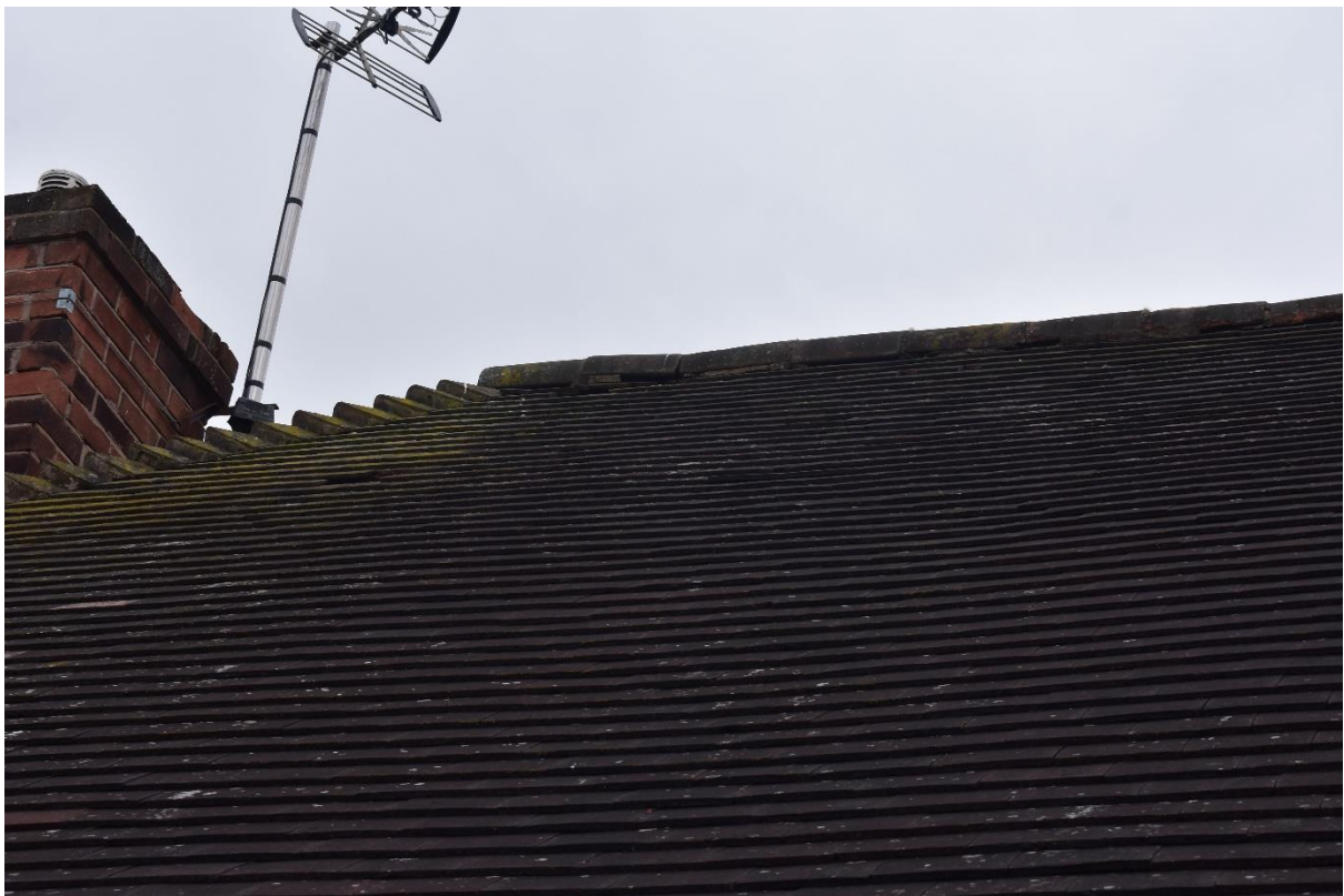
Figure 3.4: The east-facing roof of the dwelling with a lifted ridge and slipped tile.
