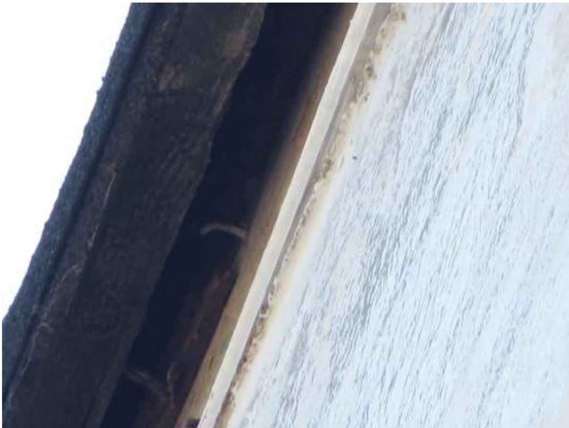
Photograph 10 – Gap between roofing felt and fascia board on Building 2, western aspect: the location of Roost 2.
