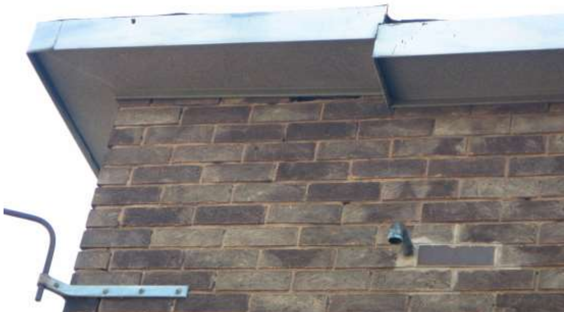
Photograph 3 - Gap in brickwork on southern aspect of Building 1.
