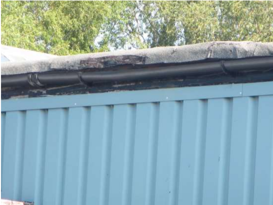
Photograph 13 – Slightly lifted roofing felt on Building 3.
