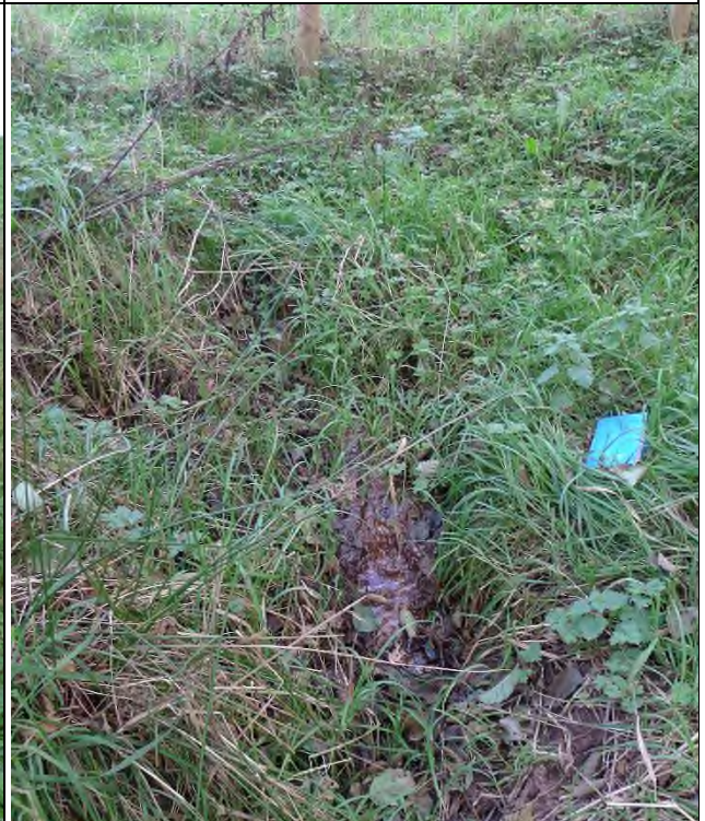
C10. Seepage line in bank of Emral Brook, 1 m below adjacent floodplain level.
