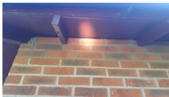
Photograph 4. Narrow gap at the top of the wall plate under the eaves.
