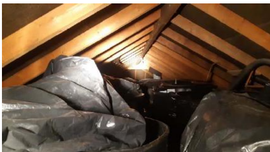
Photograph 7. Water tanks within centre of roof space, impeding access for thorough search.
