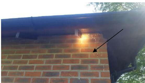
Photograph 3. Gap above the wall plate on western aspect of annexe with bird droppings and single bat dropping.
