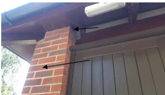
Photograph 5. North-east corner where bat dropping was noted on exterior wall, with small gap above the door.
