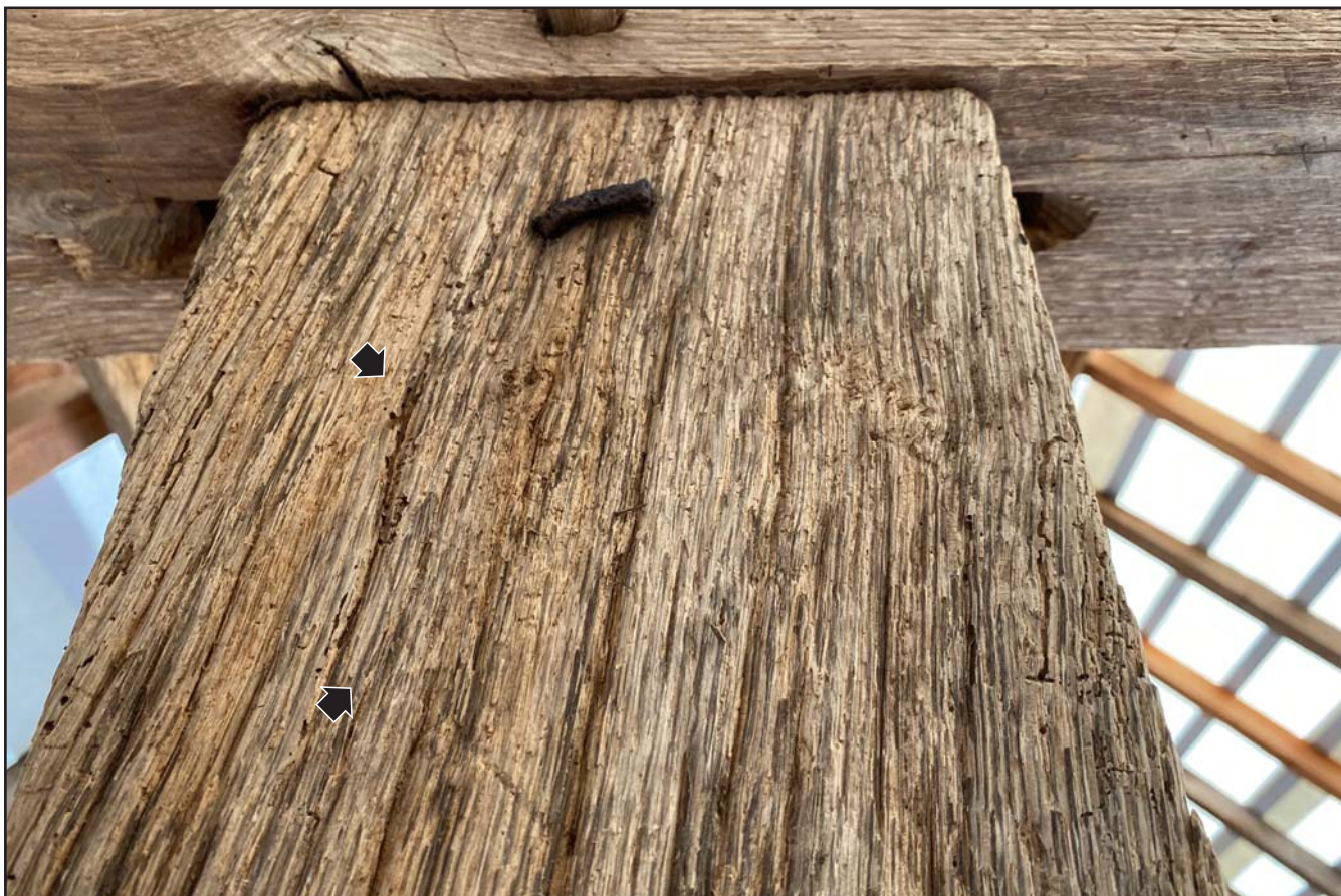
Plate 74: Possible faint Apotropaic Marks on northwest stud (near collar) of Truss 2, within Shippon 1 at Brunette Farm, Ty Broughton, Wrexham - from the east - no scale
