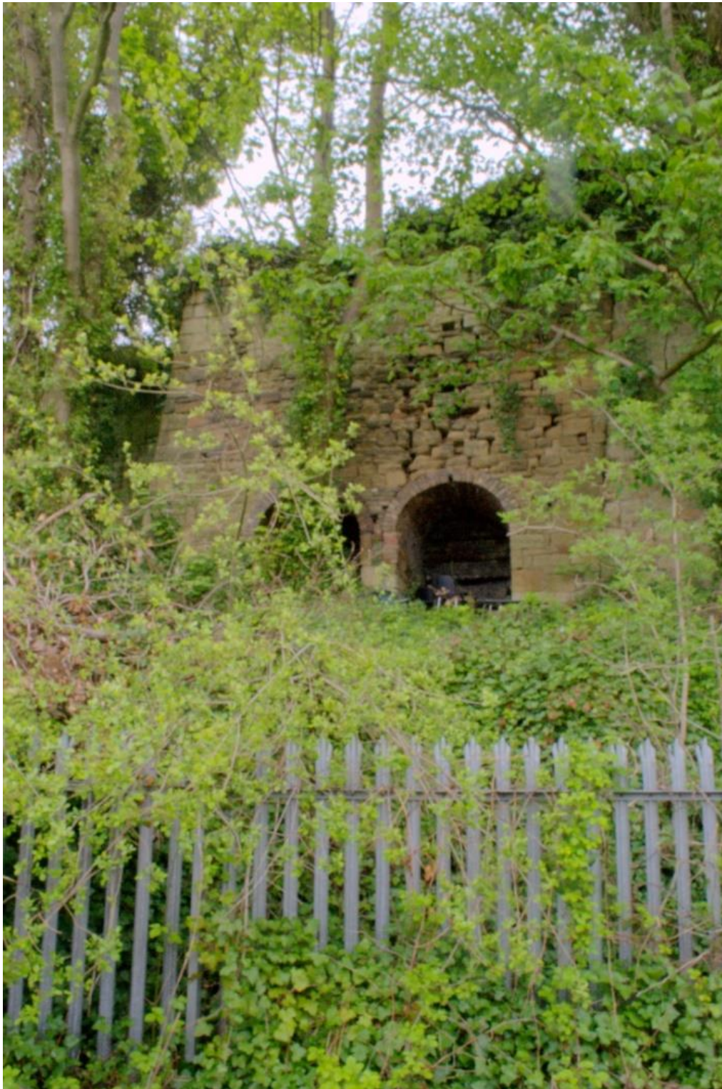
Figure 25 Furnace showing visible structural defects.
