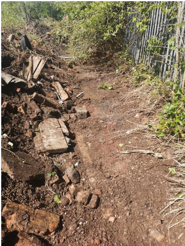
Figure 23 Area below furnaces with demolition debris and length of kerb from car parking area.
