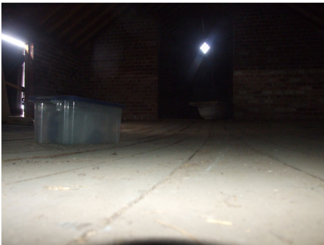
Slight sag in floor; joists and floor boards to be upgraded to comply with building regulations.
