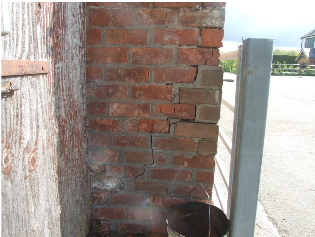
Minor damage to courtyard and left corner.
