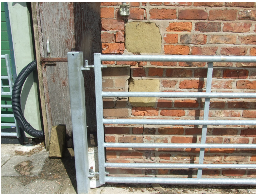
Minor damage to courtyard and left corner.
