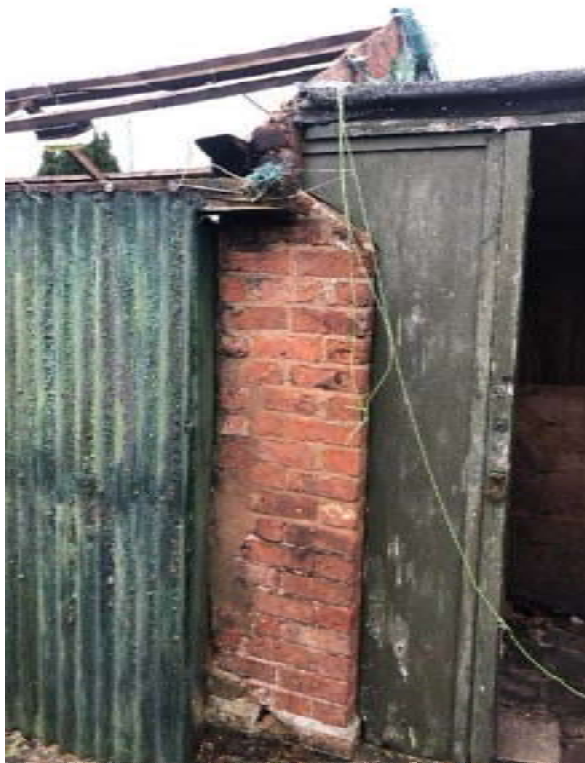
Figure 4: brick of outbuildings gable wall
