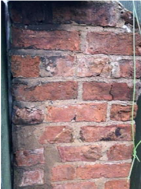
Figure 6: brick of outbuildings gable wall
