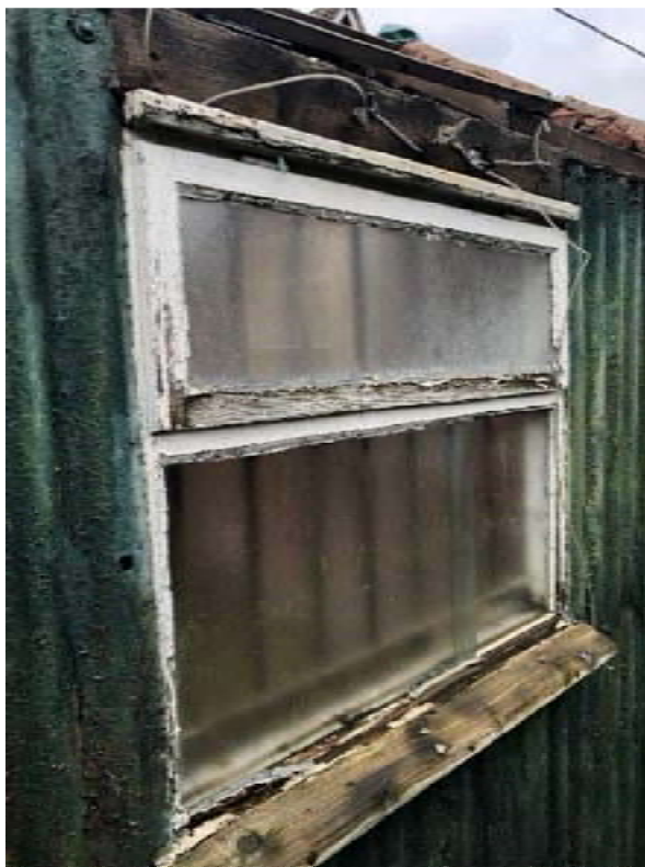
Window to outbuilding with iron bars behind
