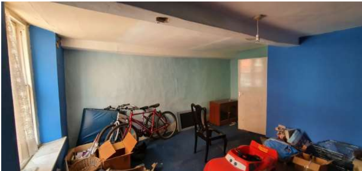
F14. Existing modern partition to be removed (right).
