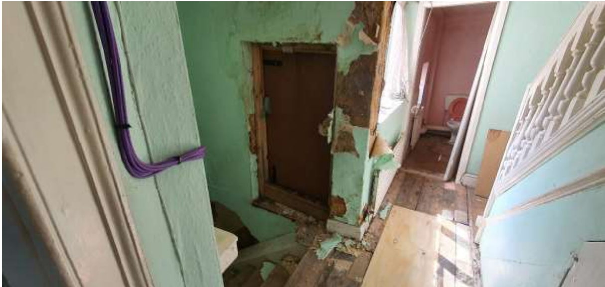
F01. Evidence of significant leaks. Proposals include for repairs to roofs.
