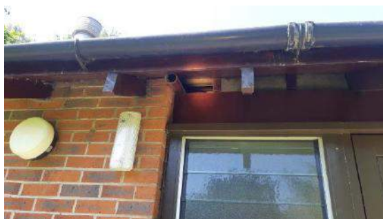
Photograph 6. Large gap where mesh is missing on eastern aspect.
