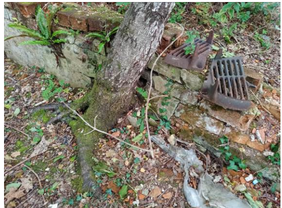
Photo 4 – Tree growing close to/within the external wall.
