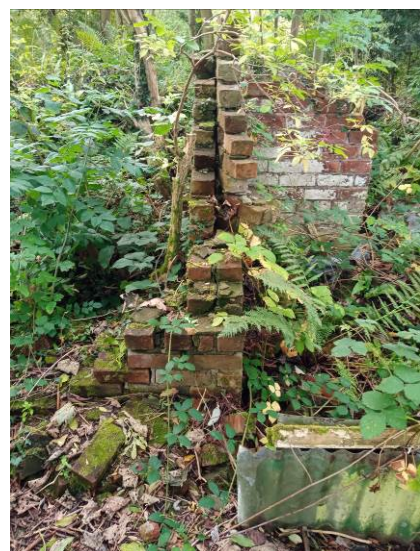
Photo 6 – Separation of solid brick wall.
