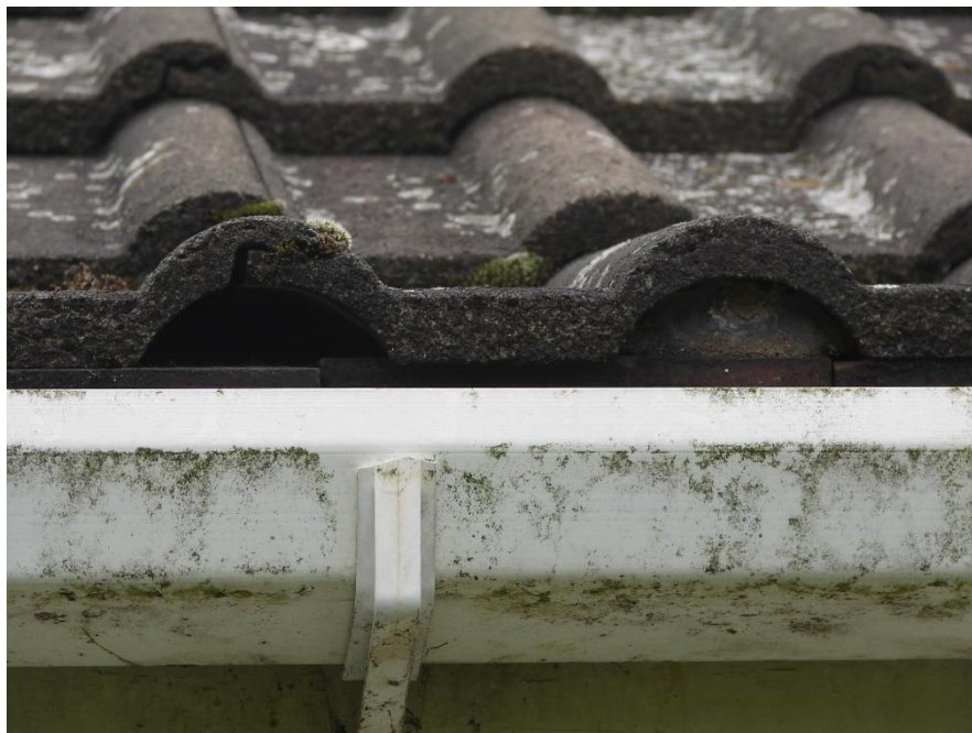
Gap in the mortar beneath the tiles at the gutter, southwest elevation.
