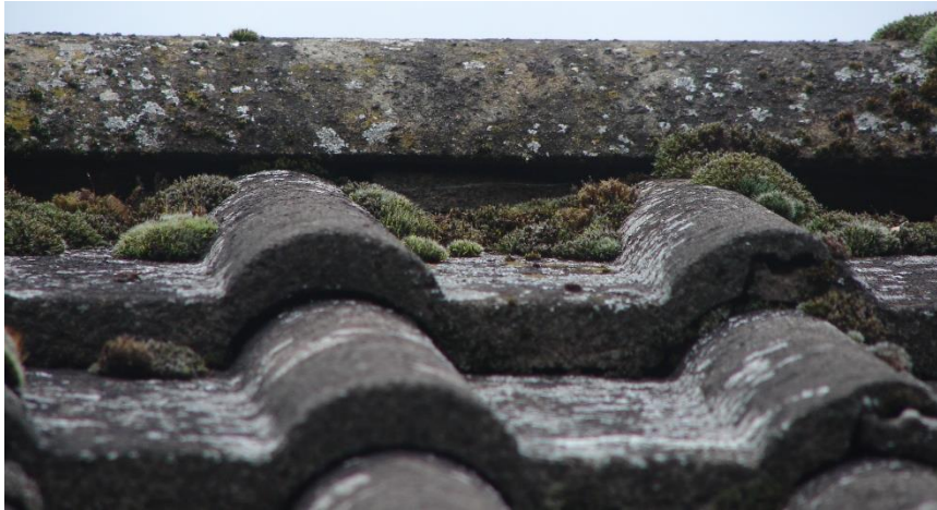
Gaps in the mortar beneath the ridge-tiles, southwest elevation.
