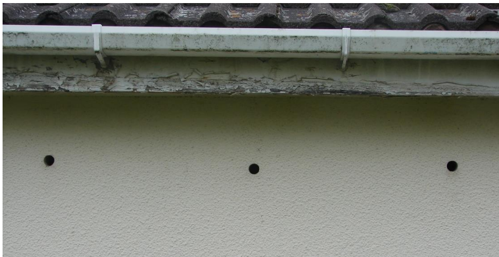
The holes shown in the photo above are believed to be built-in bird-boxes or holes drilled into the block cavity to achieve the same.
