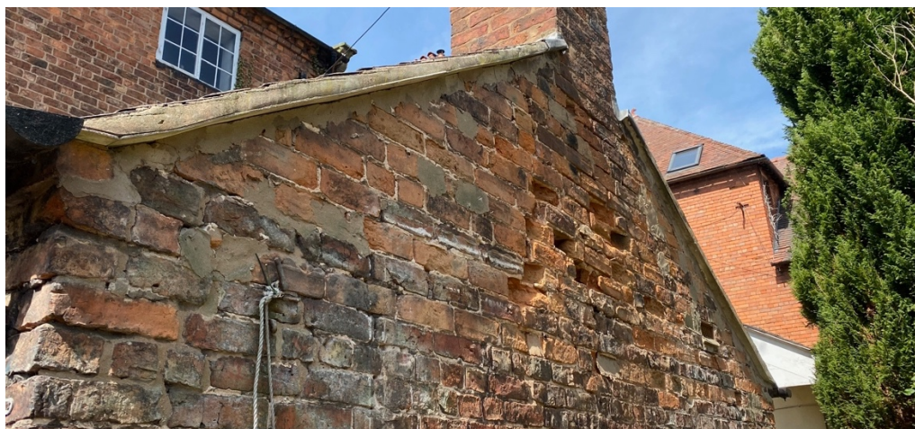
Severely eroding and poorly repaired brick to rear elevation of the existing annex
