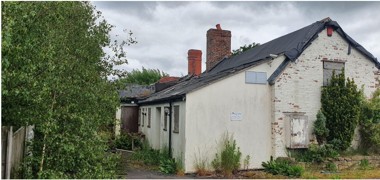
Plate 4: An image of a gap under the ridge tile.
