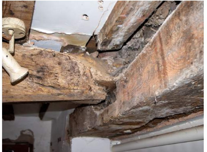
Photograph B2: (6724) Connection of the primary beam to the external wall cross beam within the kitchen. Note the splayed top face of the primary beam and notching in this beam and the cross beam.
