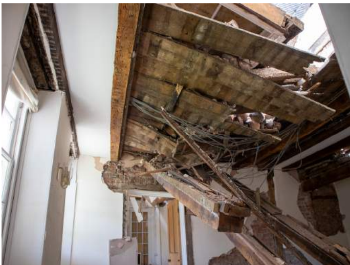
Photograph B3: (6736) View on the collapsed floor over the lounge. Note the twist on the joist but the end grain of the joists appears satisfactory. Also note the steep fall across the door head to the study.
