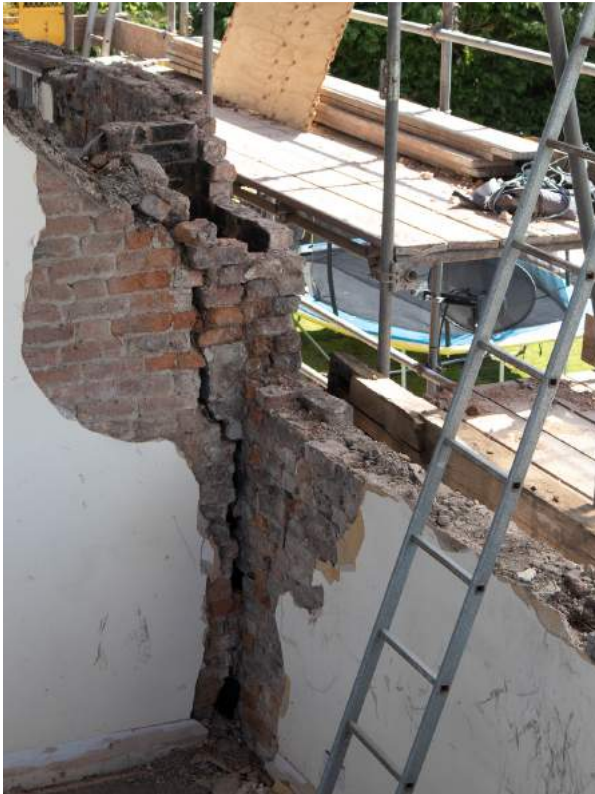
Photograph B5 (6768) showing the wide vertical fracture at the junction of the chimney stack 2 with bedroom 4. . Local rebuilding and strengthening will be required.
