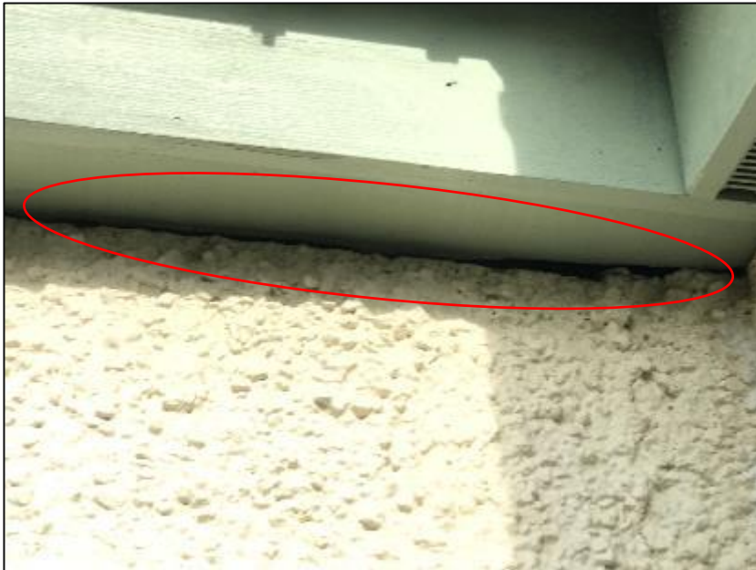
Close-up of gap along wall tops on south-eastern elevation of B1 (pictured above).
