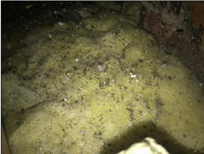
Bat droppings located within loft space of B1 (pictured above).
