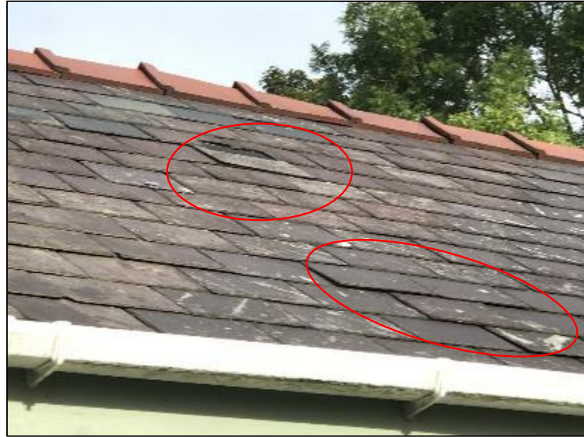
Close-up of lifted tiles on south-eastern elevation of B1 (pictured above).
