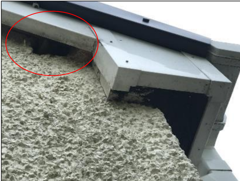
Close-up of gap along north-western gable-end of B1 (pictured above).
