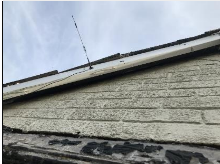
Close-up of gap behind bargeboard on south-western elevation of B2 (pictured above).
