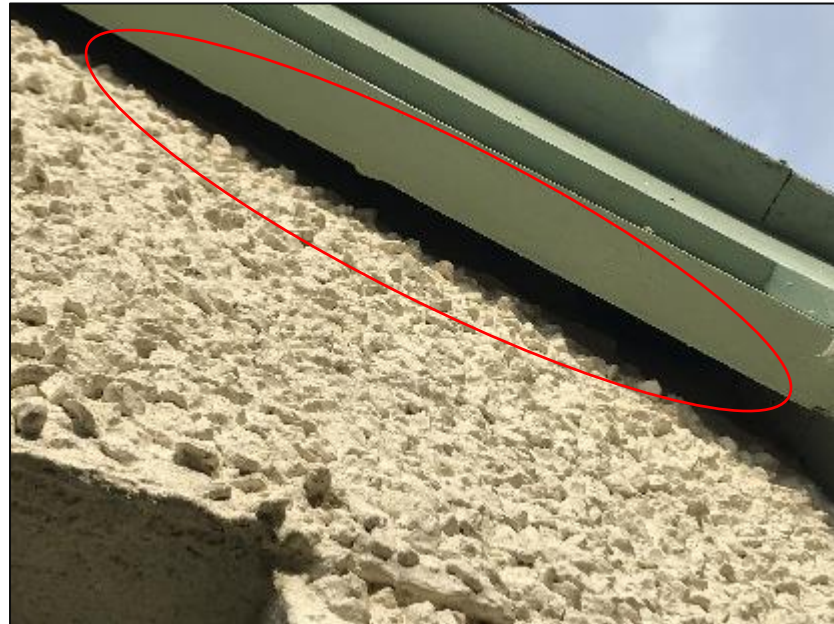
Close-up of gap behind bargeboard on south-eastern elevation of B1 (pictured above).
