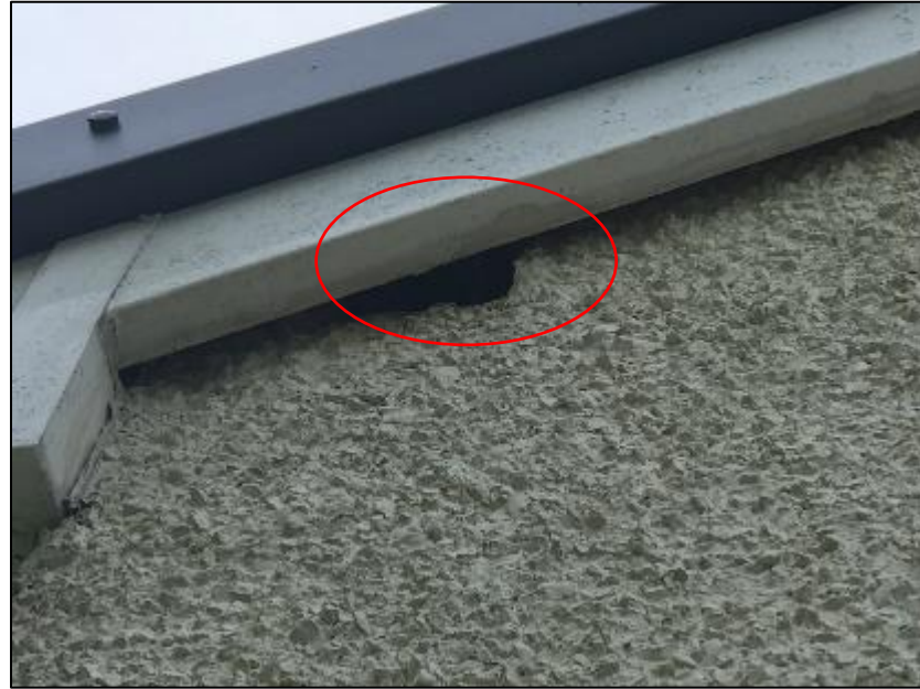
Close-up of gap on north-western gable-end of B1 (pictured above).
