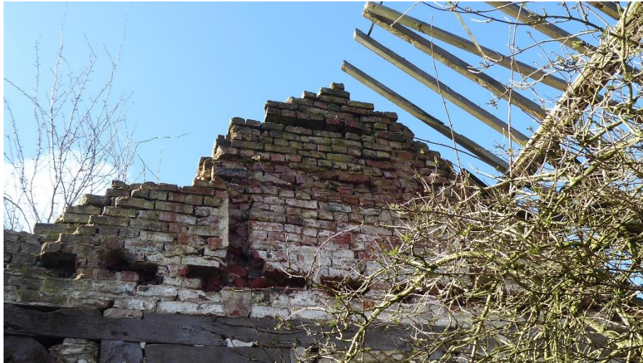
Figure 4.19. Crack and crevices in walls
