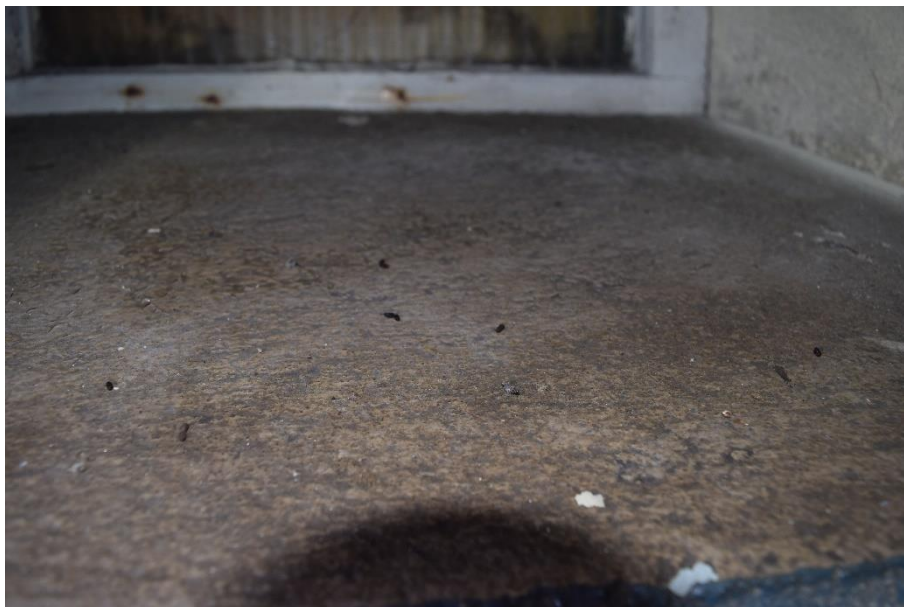
Figure 4.6. Droppings on window ledges
