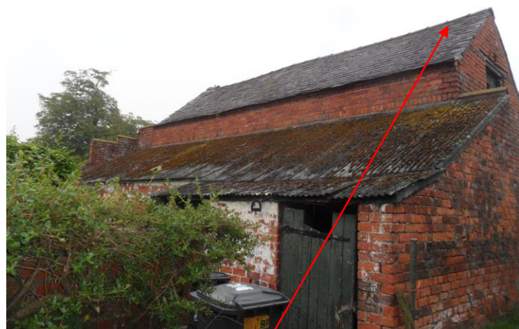
South west elevation - beneath ridge tile.
