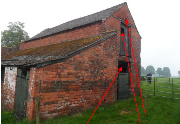
South East gable - open doors & windows and gaps in brickwork.
