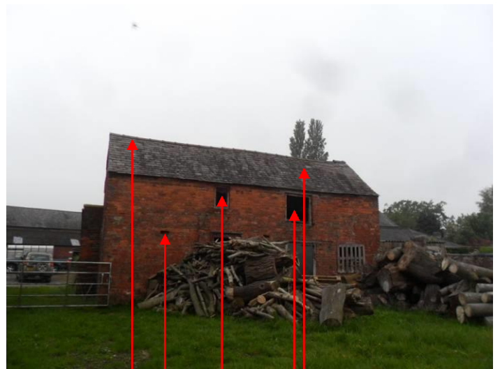
North east elevation - Beneath ridge tiles/ displaced roof slates, open doors & windows and gaps in brickwork.
