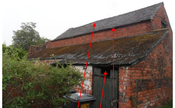
South west elevation - Beneath ridge tiles/ displaced roof slates and gaps around doors.
