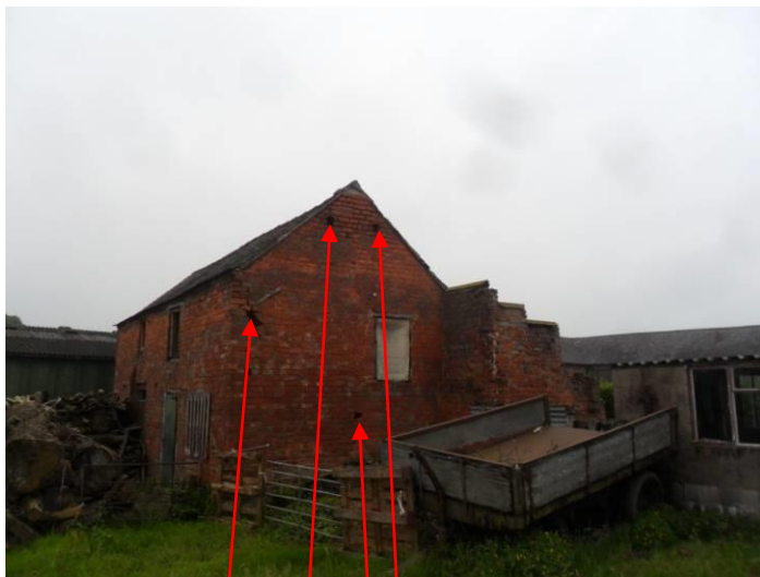
North west gable - Gaps / stress fractures in brickwork
