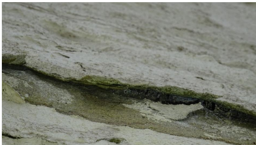
Figure 4.6. Crack in external render
