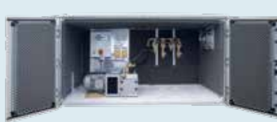
Concrete external cabinet
