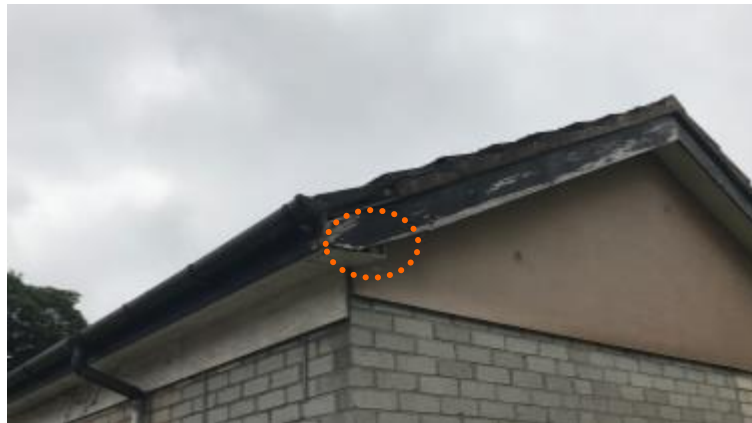
Figure 5.4 - Visual Aid - Emergence location at a gap in the northern end of the western gable soffit from which one Common Pipistrelle emerged during dusk survey 1 and two Common Pipistrelle emerged during dusk survey 2
