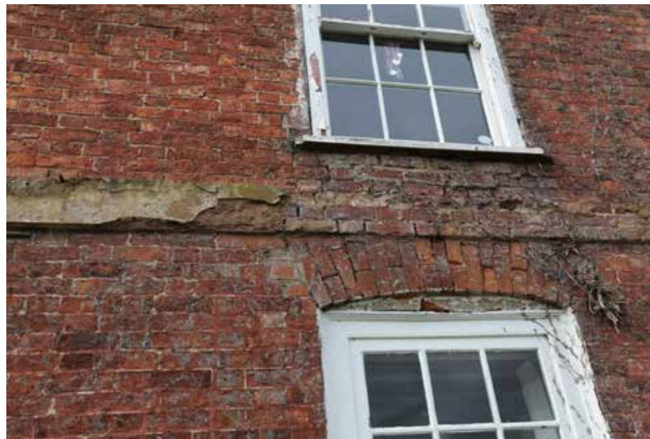
Plate 5 above: The raised bands between the floors comprised three courses of projecting brickwork and were finished in stucco. The brickwork is in very poor condition and the stucco will need to be reinstated, as originally intended. This image shows the Dining Room window with its segmental rubbed brick arch and the moulded architrave to the sash window, as originally designed. The sash window above is modern and incorporates a projecting timber cill, which is incorrect for the period. It also has 'horns' and has no architrave. To the left of the Dining Room window we can see evidence of the original 'tuck-pointed' joints which provided a high degree of refinement. This has been affected by subsequent repointing and the poor condition of the masonry, a large part of which is the result of rampant ivy.
