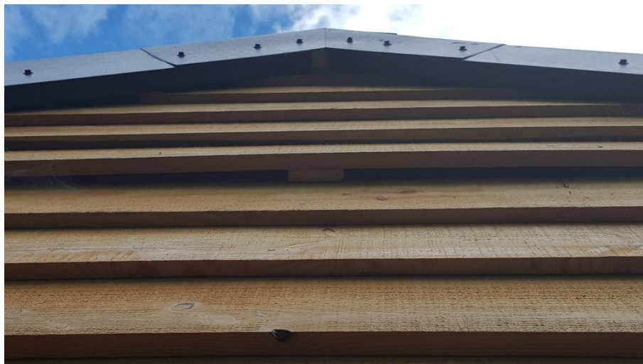
Figure 6.2. Artificially raised timber cladding
