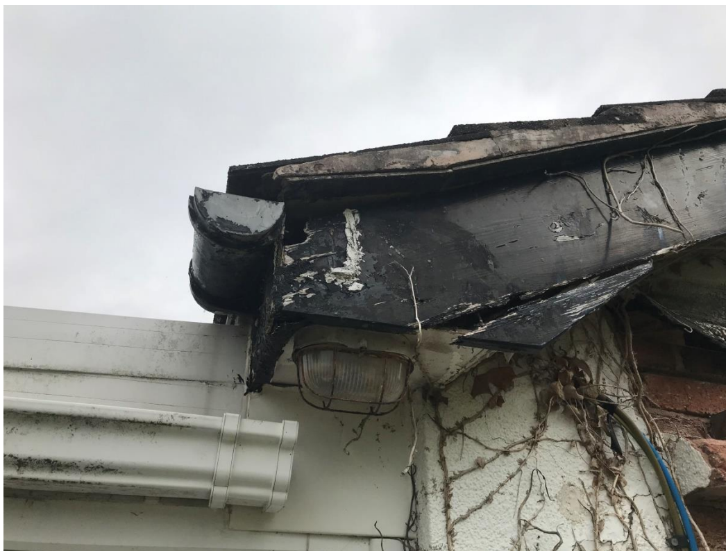
Plate 7 – Gap in the soffit
