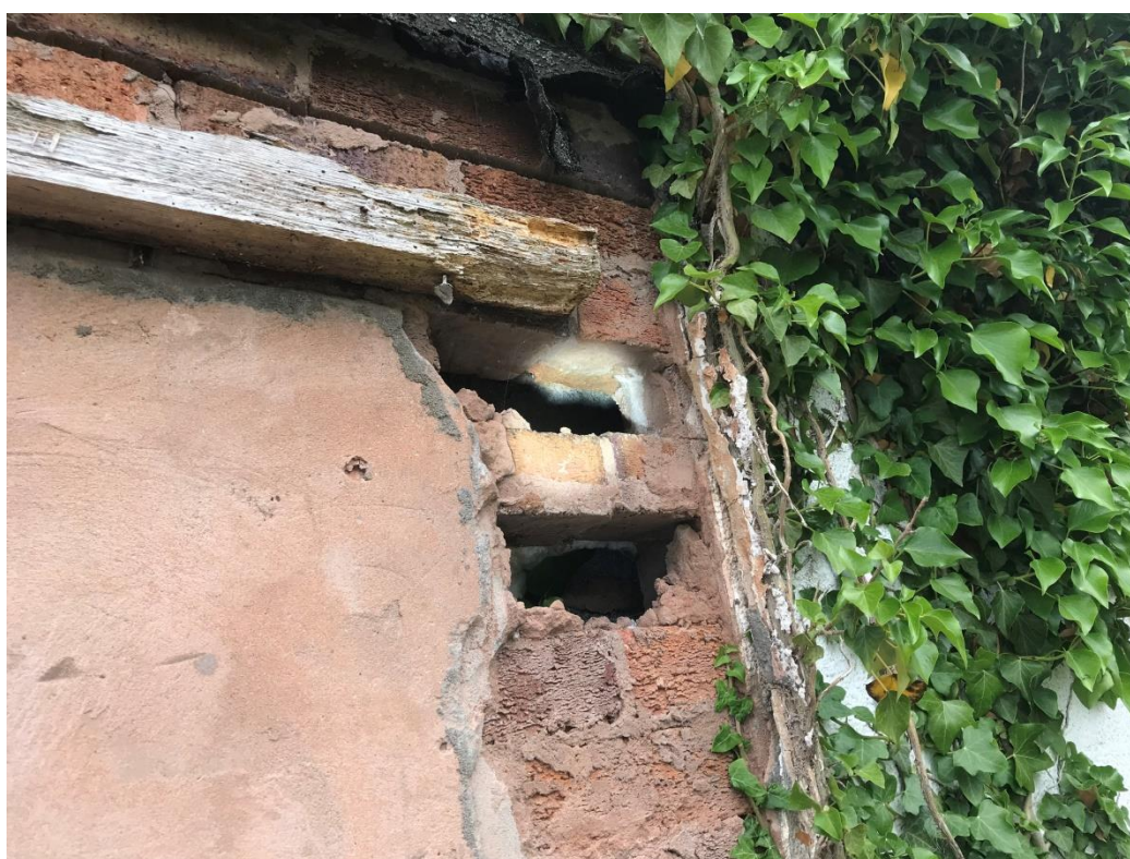
Plate 6 – Gaps in brickwork leading into the cavity
