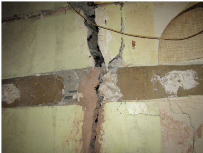
Photo 8: Shear cracks in supporting wall on first floor of building.
