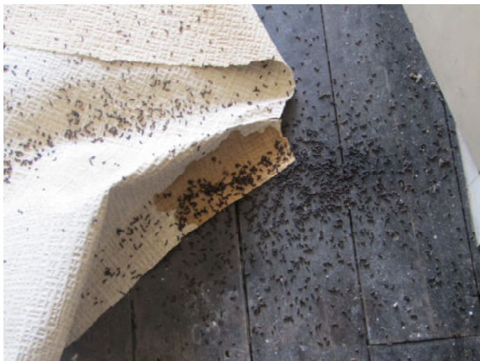
Photo 6: Closer detail of LHS bat droppings on landing of first floor.
