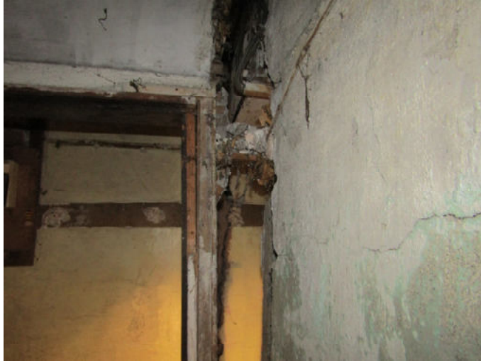
Photo 7: The doorframe originally was flush with the wall, but the supporting wall has sheared and movement has created a huge gap in first floor of building.
