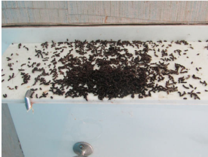
Photo 4: Lesser Horseshoe bat droppings on shelf above sink in bedroom.
