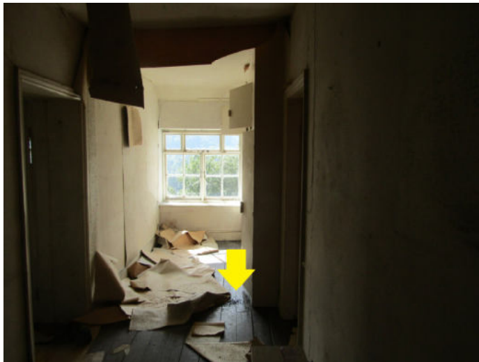
Photo 5: Bat droppings on landing of first floor near South elevation.
