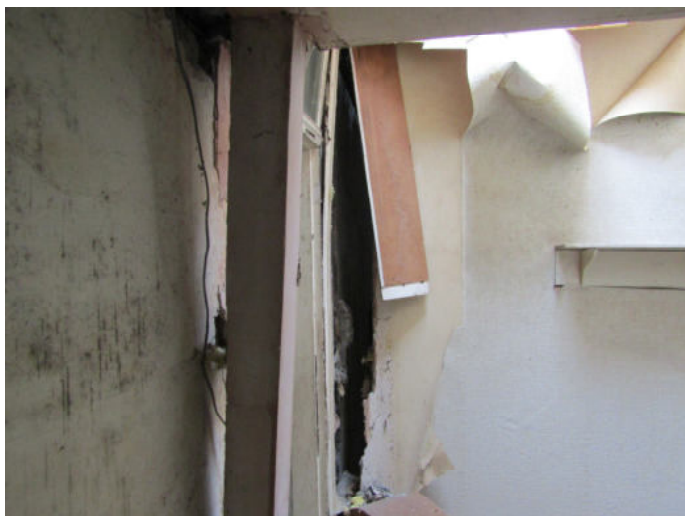
Photo 9 Shear cracks in supporting wall on first floor of building.
