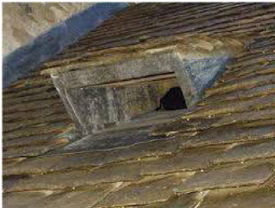
Figure 14: Example of LHS covered fly in access in roof.
