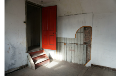
DAMAGAGED PARTITAL WALLING PANELING TO BE REMOVED
