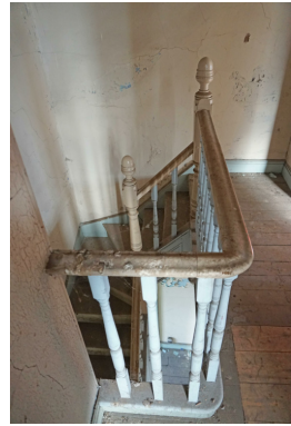
DAMAGED STAIRWELL TO BE REMOVED, FEATURES, NEWELS AND SPINDLES ETC TO BE ASSESSED FOR REUSE
