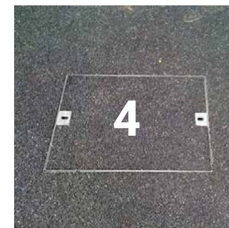
Recessed manhole covers
