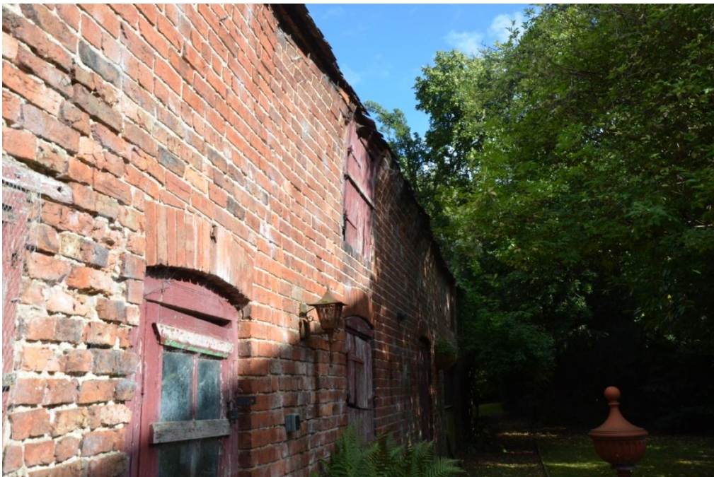
Photo 2 - Front elevation of Higher Oak Barn showing bowing at the top of the external wall beneath the eaves prior to structural repair works.
