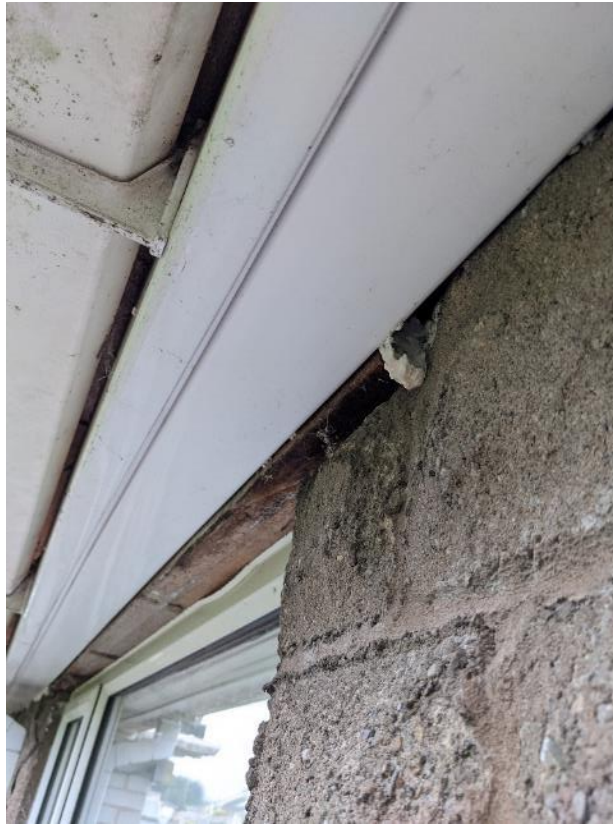
FIGURE 4.4: SPARROW ENTRY POINT UNDERNEATH BARGEBOARD ON NORTHWESTERN CORNER
