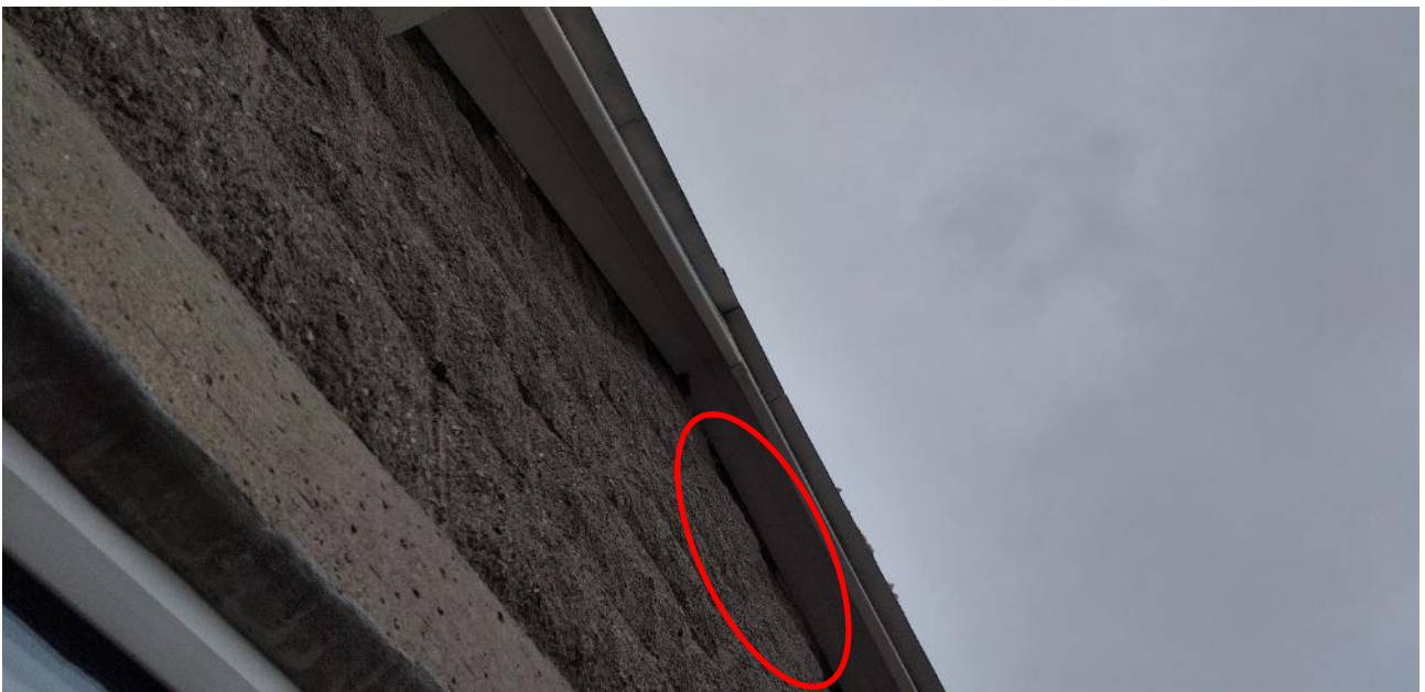
FIGURE 4.5: SPARROW ENTRY POINT BEHIND SOFFITS ON SOUTHWESTERN GABLE
