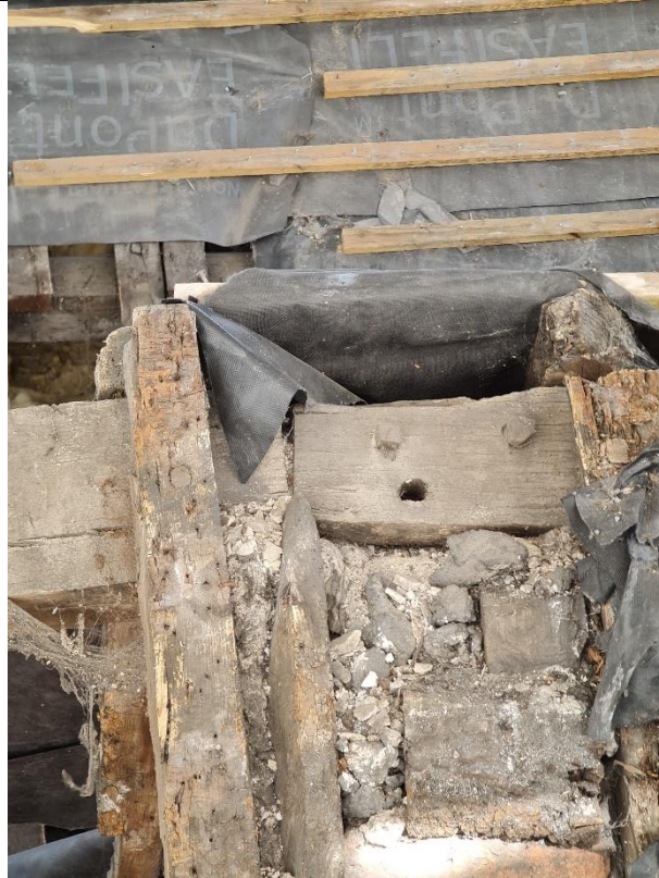
Ridge beam not supported
