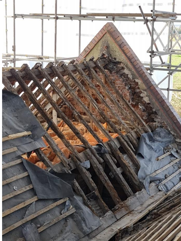
Loss of section to rafters
