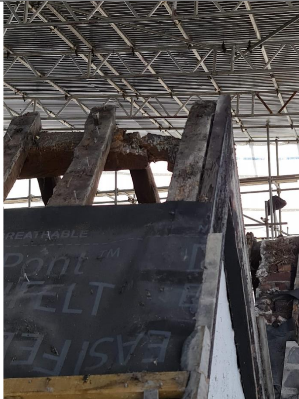
Failure of ridge beam
