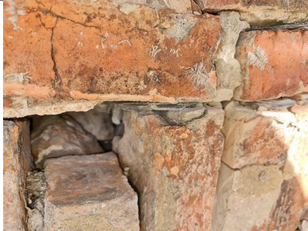
Void through to timber lintel behind
