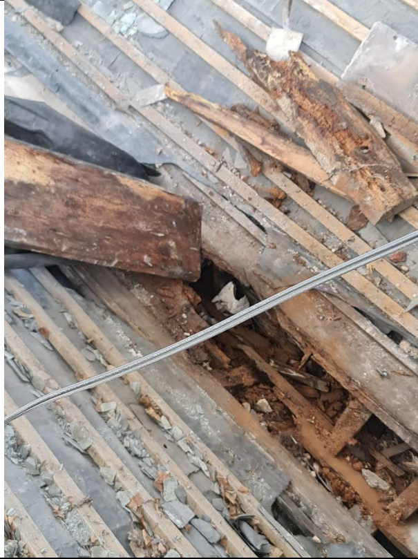
Severe rot to valley
