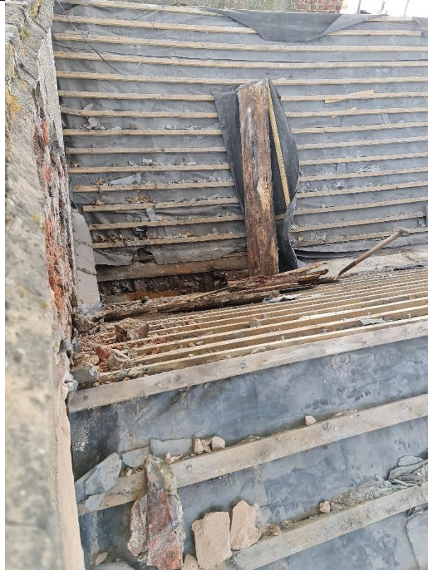
Rot to valley gutter
