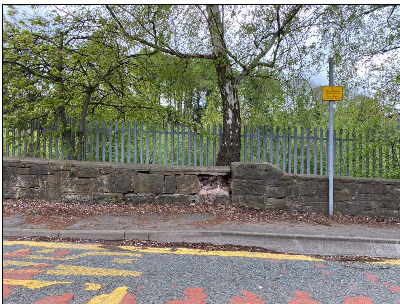
P5 – T5 displacing boundary wall
