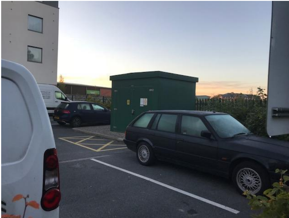
PLATE 3: ELECTRICITY SUBSTATION LOCATED IN THE NORTH OF THE SITE
