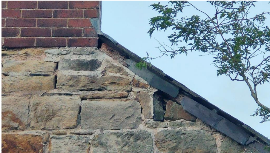
Figure 4.6. Damage to northern gable end
