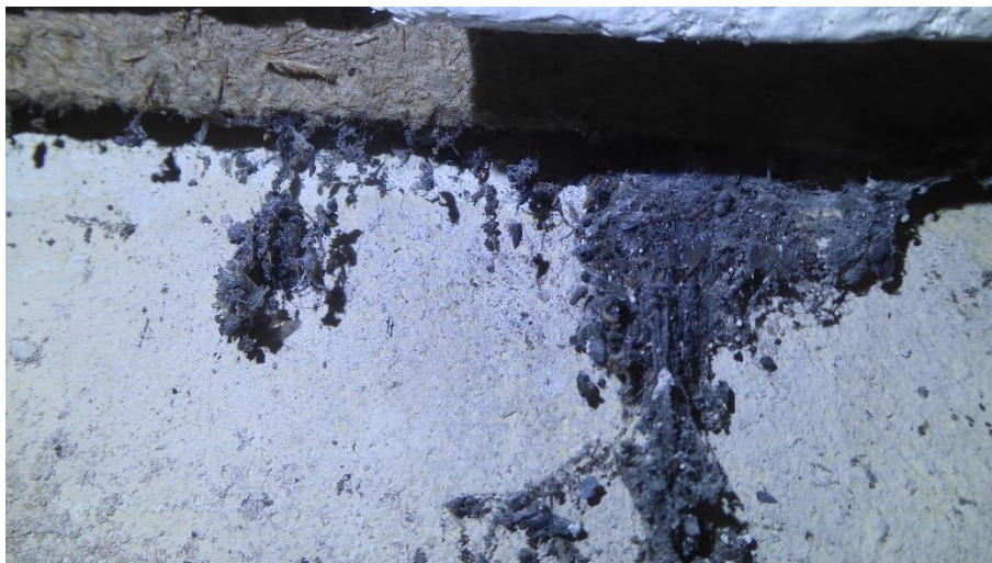
Figure 4.5. Droppings caught in cobwebs dropping from ceiling holes
