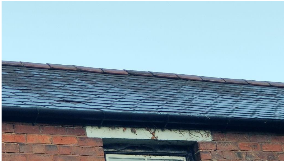
Figure 4.7. Gap beneath ridge tile
