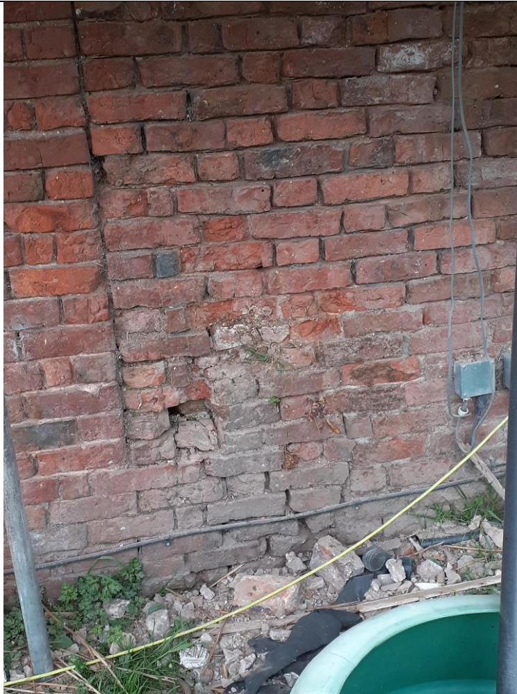
Decayed masonry not tied in.
