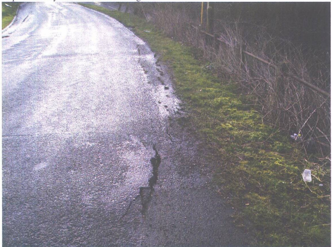
Evidence of slope instability on south eastern site boundary
