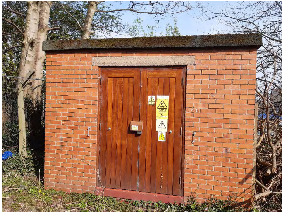
Photograph 5- Facing north showing the substation.
