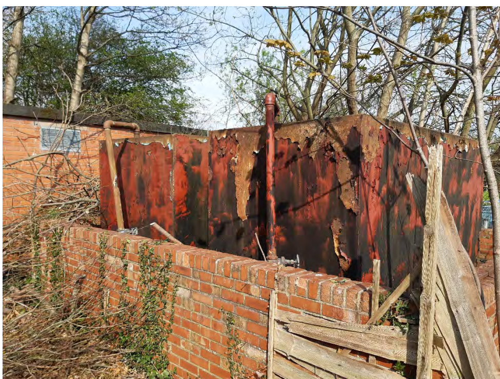
Photograph 8- Showing tanks on site.
