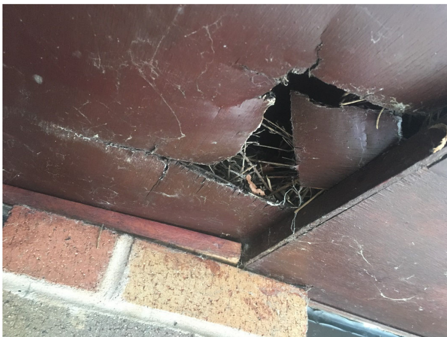
Plate 5: Damaged soffit with nesting material within soffit box
