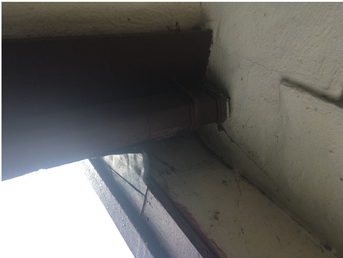
Plate 8: Gap in flashing were roofs adjoin
