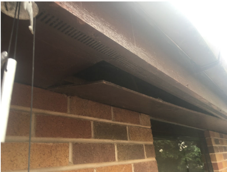
Plate 4: Example of damaged soffit
