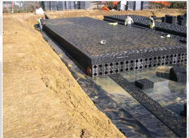
350 mm central access channel with multiple outlets
