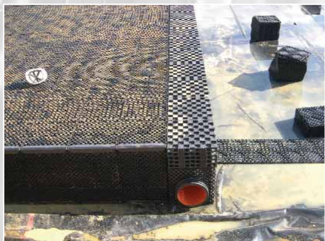
350 mm access channel through system
