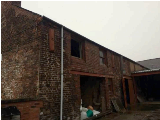
Plate 2: Building 13 showing broken window
