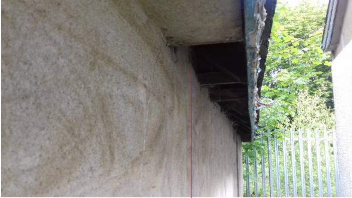
Gaps in soffit of B2
