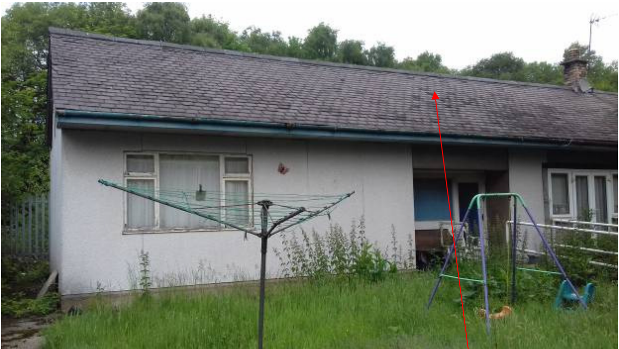
Bungalow (B1) front elevation showing missing tiles/loose/lifted slates
