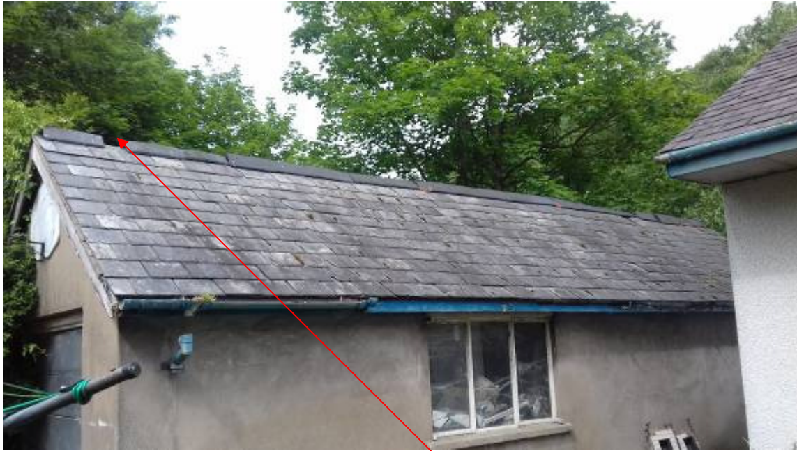
Garage (B2) showing loose/lifted tiles and missing ridge tiles with gaps at wall plate level
