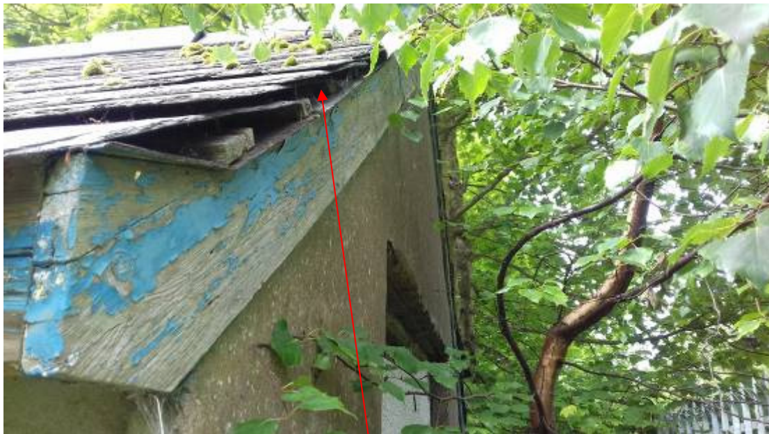
Gaps in the roof verge within B2
